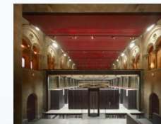
Marenostrum, Barcelona Supercomputing Centre (Barcelona)
